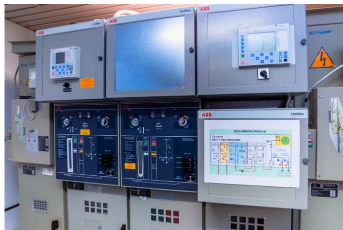
Figure 3: Medium voltage switchgear installed at ACEA's test field, with instruments for the selection of MV lines failed segments
